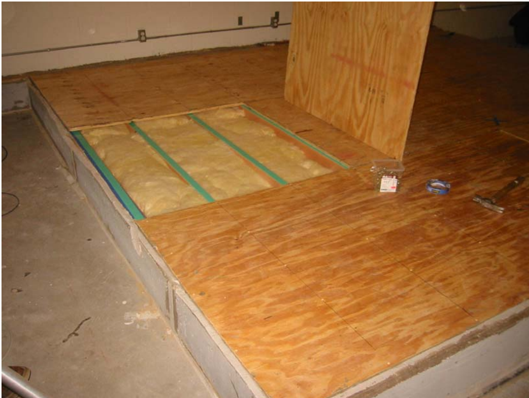
Figure 1: Floor side of floor / ceiling; opened to reveal Norlin CST™ joist tape
